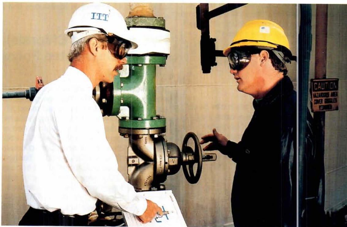
Tefzel ® ETFE lined, Kynar ® PVDF coated Dia-Flo Diaphragm Valve shown in specialty chemical manufacturing plant on 35% HCl line.
