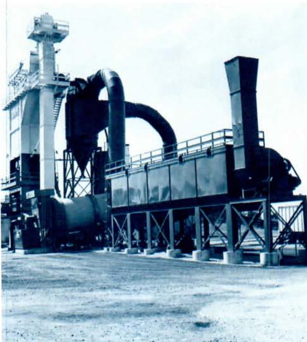
This asphalt fabric filter type dust collector uses Screw Conveyor flighting in the hoppers which return collected fines to the mix.
