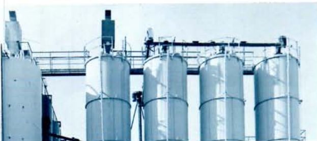
Partial view of a large outdoor installation employing Screw-Lifts to elevate material to fill storage silos.
