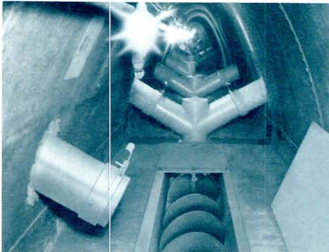
This Screw Conveyor in a tunnel installation illustrates the compact arrangement possible when space is at a premium.
